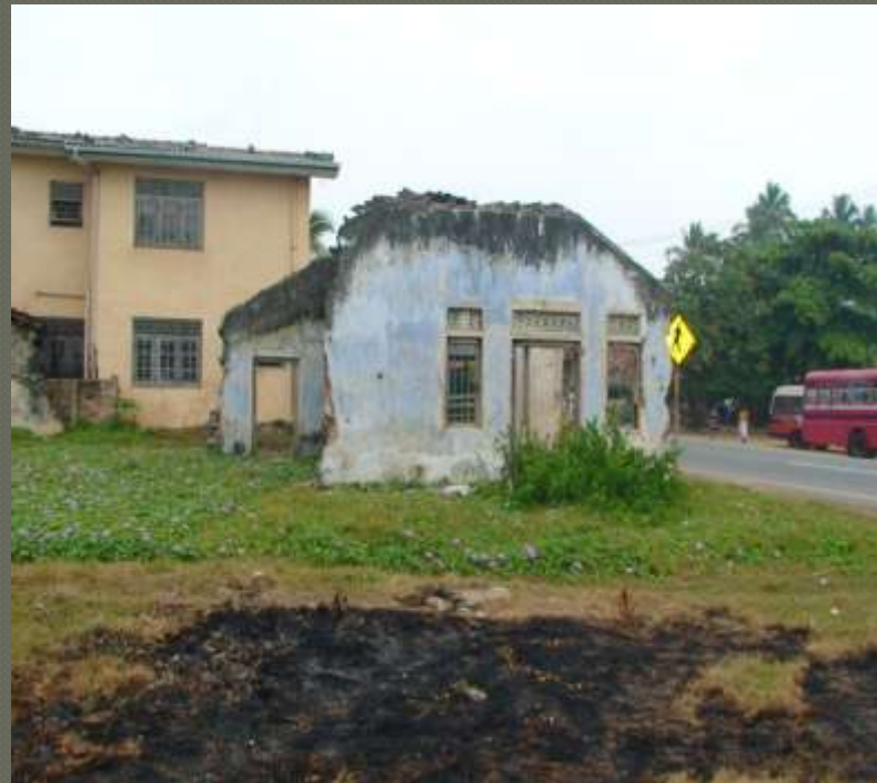
Tsunami hits the house
